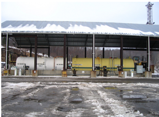
Aboveground fuel storage tanks at a Tilcon New York, Inc. facility.
